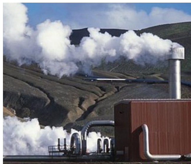
Geothermal power plant
